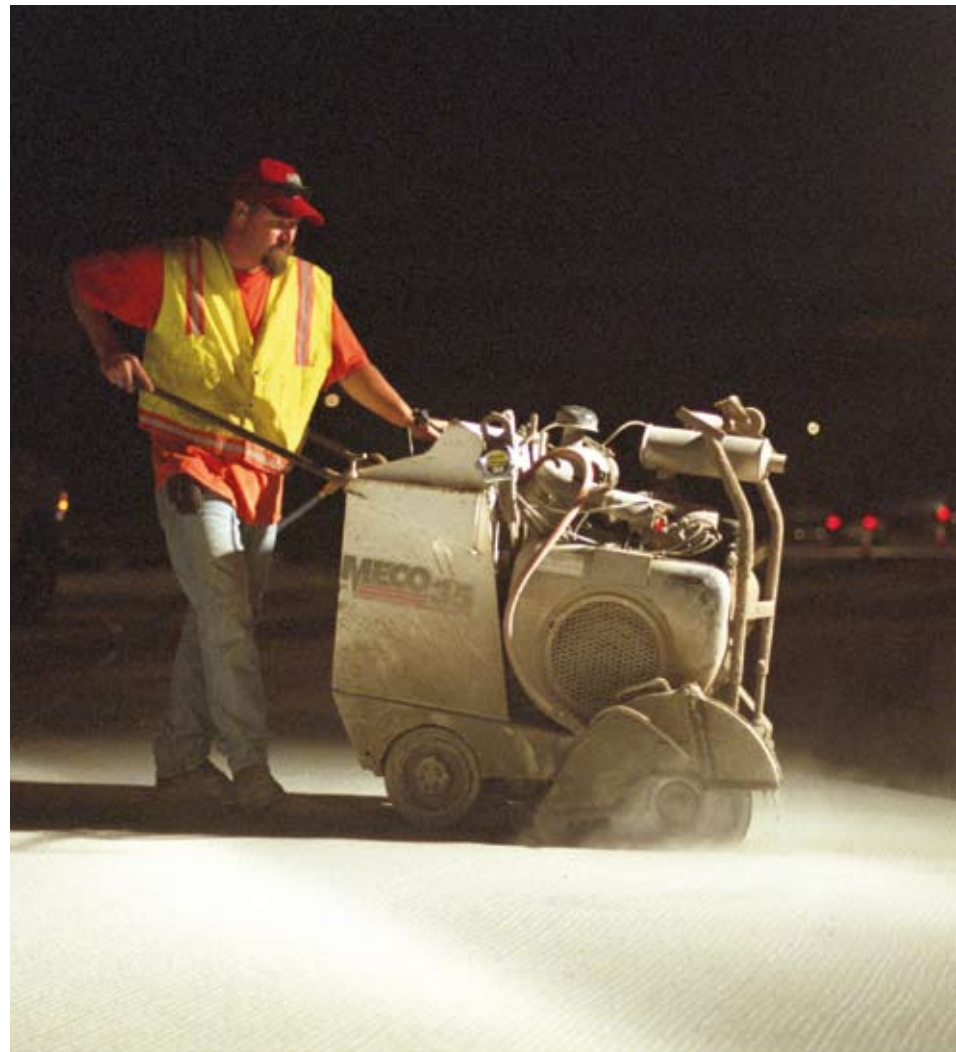
Contractors are permitted to saw cut the perimeter of the damaged slabs up to two days before removal so the sawing operation will not hinder the fast-paced replacement process.
