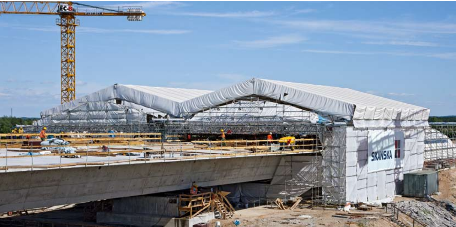
Two movable weather protection roofs span two incremental launching facilities for the construction of a bridge superstructure near Grudziadz in Poland. Photo Credit: PERI GmbH.
