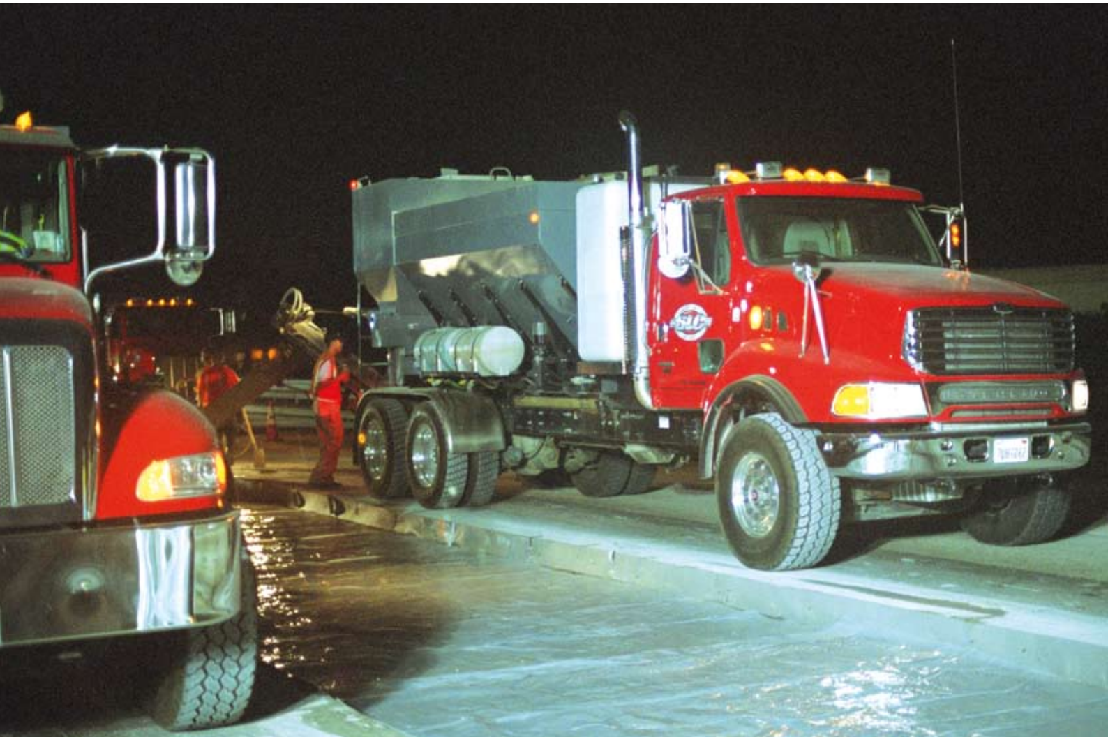
As is typical for Caltrans projects, the repairs had to be performed during a night shift to minimise lane closures.
