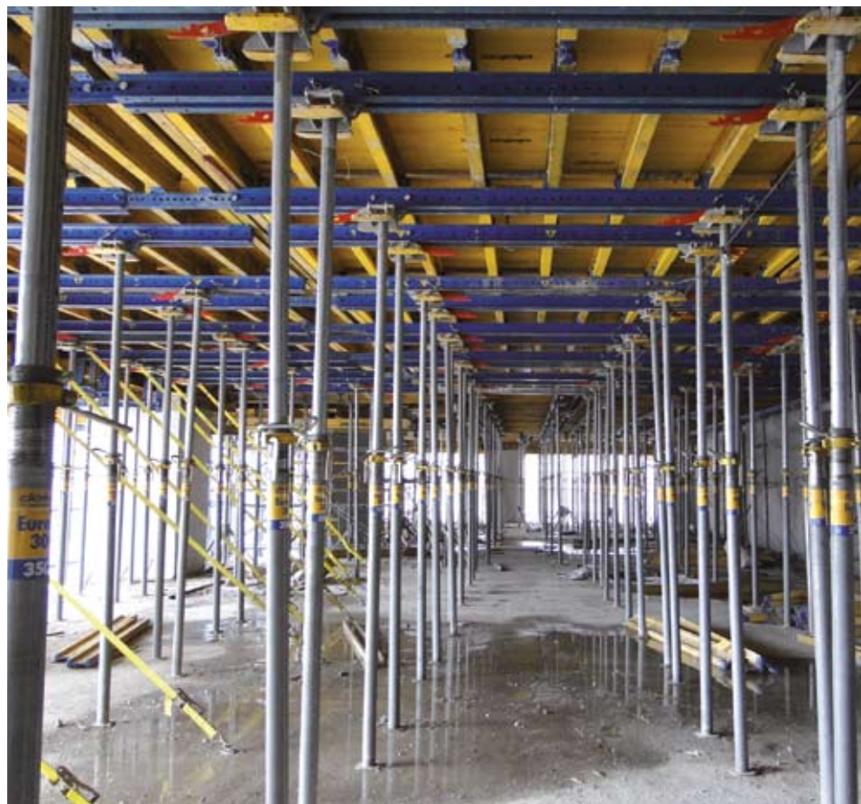
Completely preassembled Dokamatic-Tables are in use for the 60 floor high commercial and residential building.
