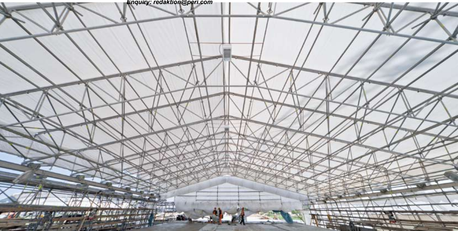
Roofing for the scaffold construction is provided through a Keder system whereby the integrated sheeting offers the best protection against wind and weather. Photo Credit: PERI GmbH.
