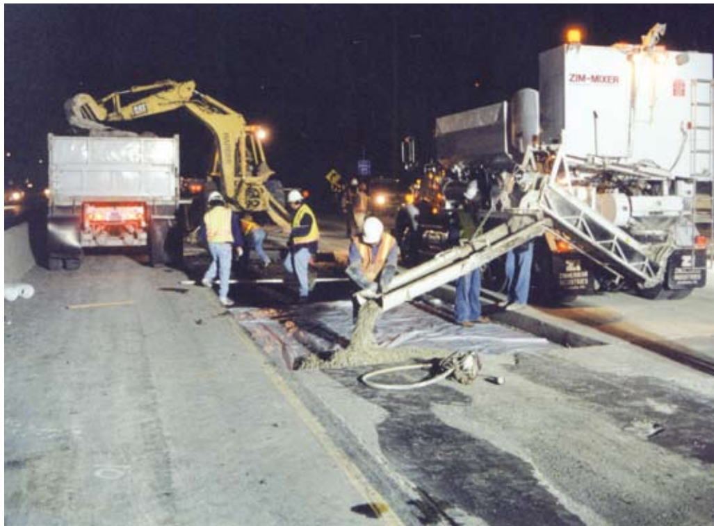
To ensure the advantage of replacing individual slabs is that using rapid-strength concrete repairs can be achieved overnight and lanes opened to traffic in time for the morning commute.
