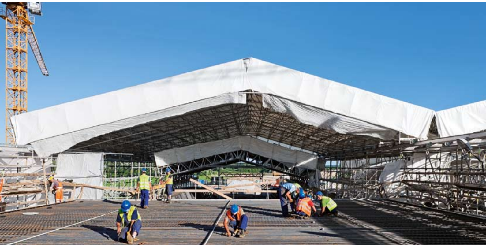
For the reinforcement and concreting work, the weather protection roof is pushed over the permanently installed reinforcement tent. All required materials can then be craned in without any problems. Photo Credit: PERI GmbH.
