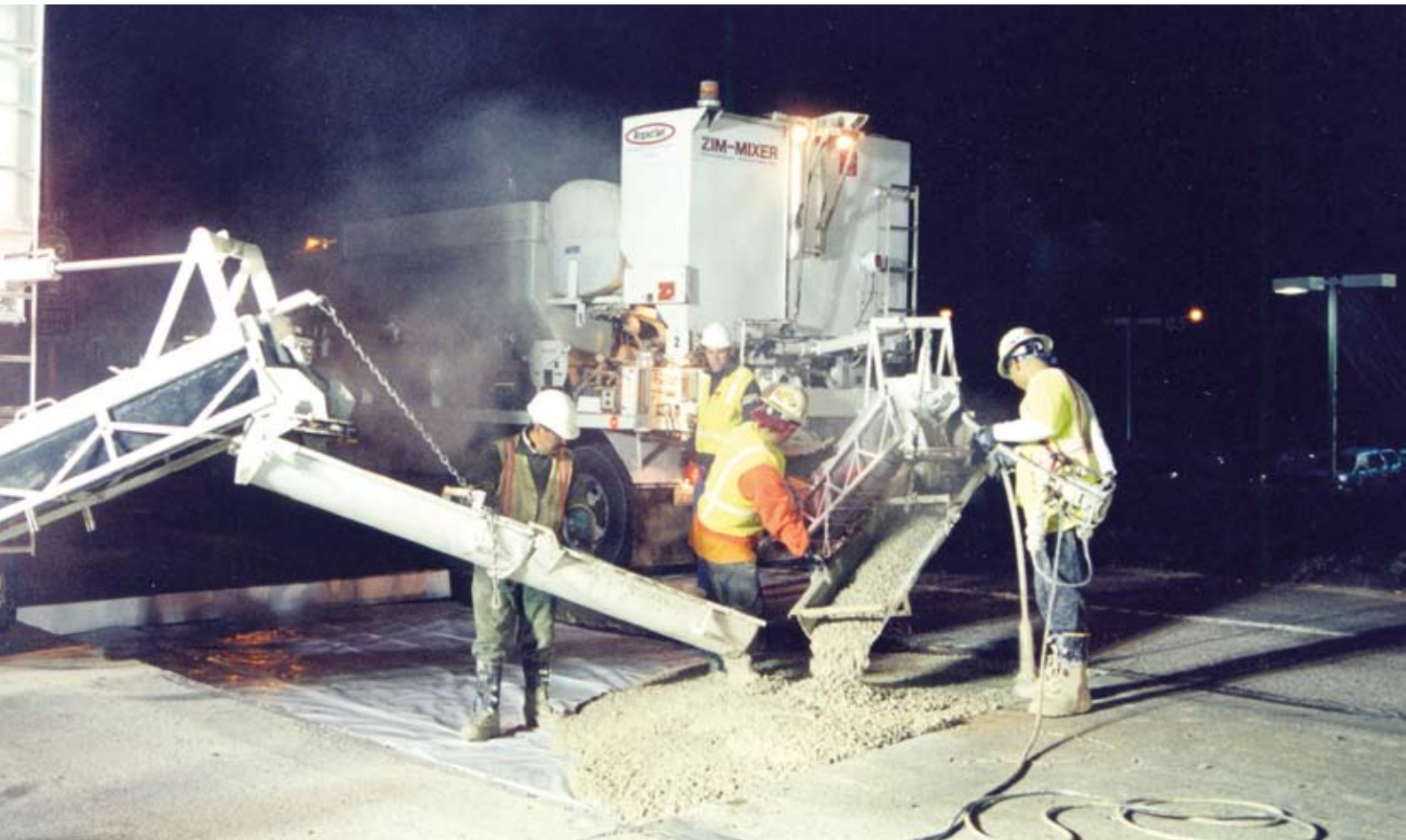
The concrete for the project, produced in volumetric mixers, used Rapid Set® cement, a fast-hardening hydraulic cement made by CTS Cement Manufacturing Corporation.
