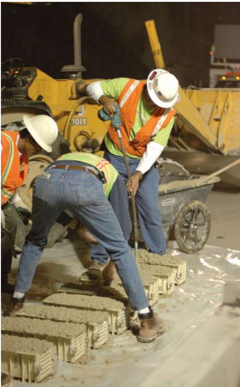
Twining's mobile testing lab conducts beam tests on the jobsite to verify and seven-day flexural strength values.
