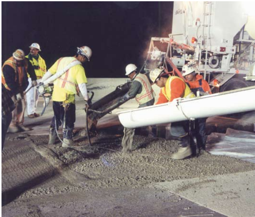
Volumetric mixers facilitate concrete production onsite rather than in transit, which is critical given the fast setting time of the concrete.
