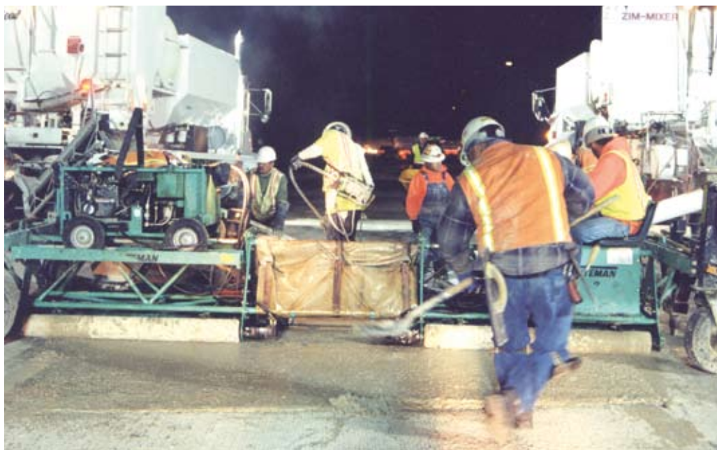
To ensure that everyone involved on pavement projects understands how to work with the unique properties of rapid-strength concrete, Caltrans requires all personnel to attend a formal Just In Time Training (JITT) program.
